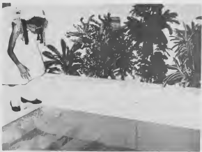
FINISHED TILE work for the Baptistry was laid by members of the church. It is behind the lecter. OBRA DI azulejo pa e bautisterio a wordo pao door di miembronan. E ta keda tras di e preekstoel.
